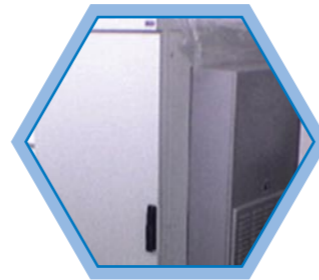
Outdoor Air-Con Rack
